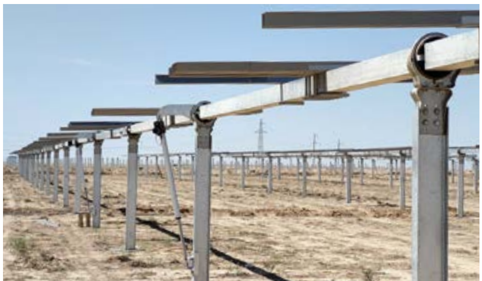
Trina Tracker installed in Habei, China, 400 MW
