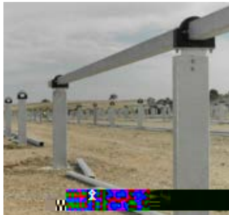
Spherical bearings installed in Zuera 11 MW, Zaragoza
